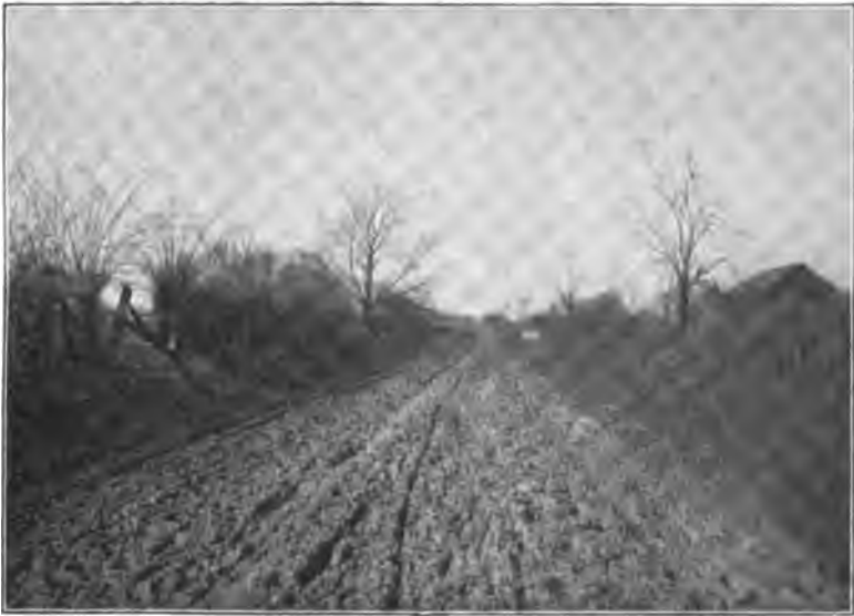
Neshanic road, Somerset Co., before improvement.
